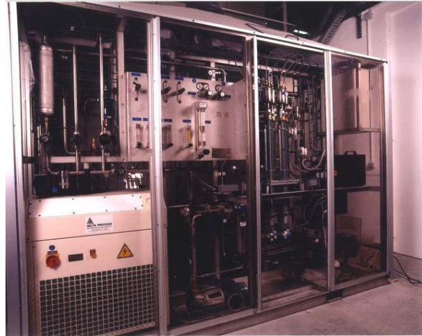
First automated system, installed at Moissy-Cramayel (France) for ensuring Kr and Xe very high-level purification. A whole factory building is now dedicated to such rare gas purification and the process is fully computer-control, working 24/24. A similar factory has been put up in Germany
